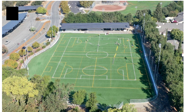
AFTER THE SYNTHETIC TURF IS IN PLACE WORKERS GET FIELD 2 NEAR COMPLETION
